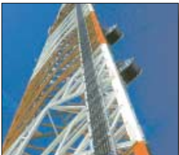
Towers —Monitor obstruction lighting failures to increase safety and avoid fines by the FAA.
